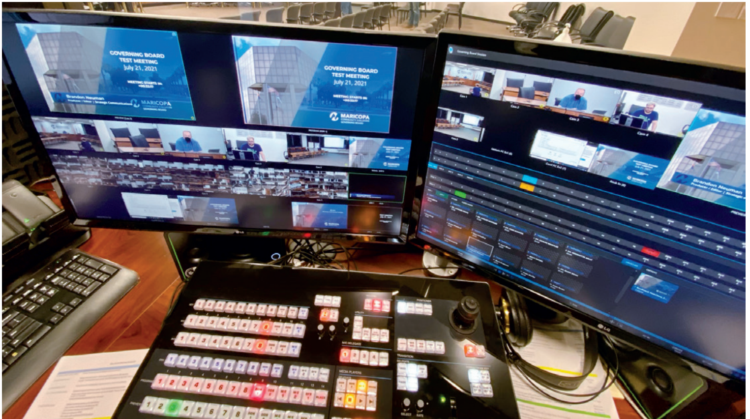
From the adjacent control room, the MCCCC operator is able to monitor and operate the DTP system, facilitate streaming and recording, as well as manage feeds and AV content availability for the broadcasters.
