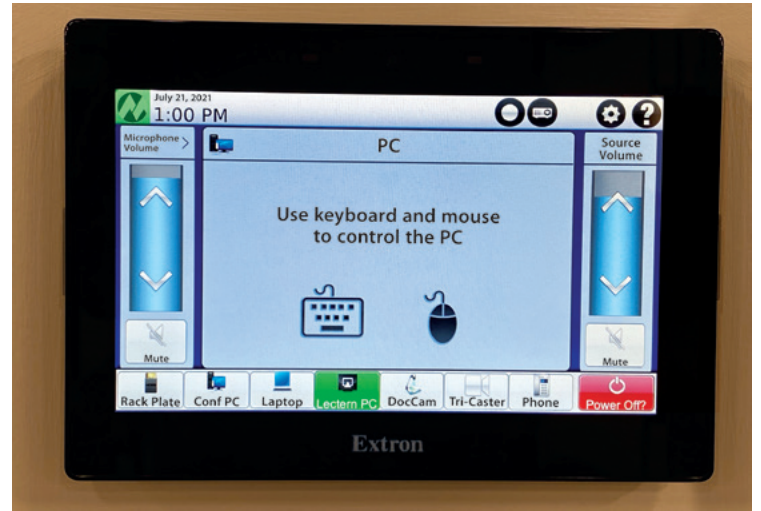
Presenters operate the AV system using the TLP Pro 725M TouchLink® Pro touch panel mounted on a side wall of the board room.
