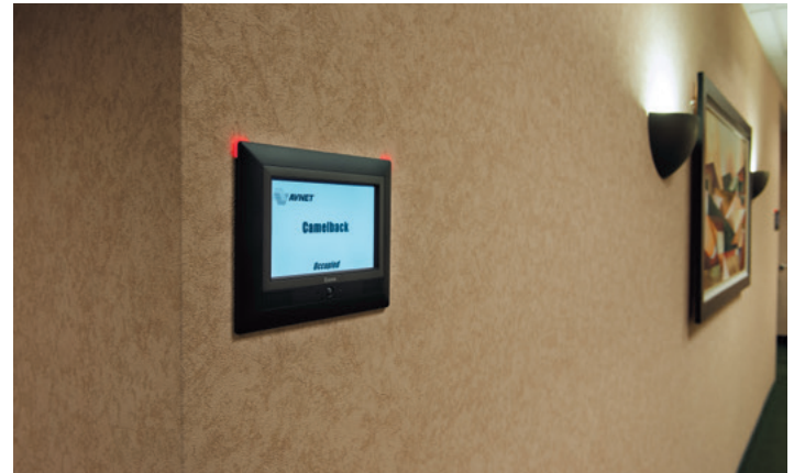
Touchpanels at room entrances are configured to indicate space availability.
