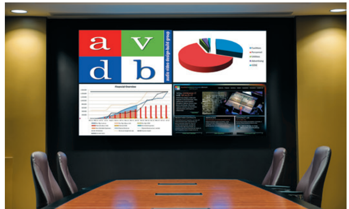
The Phoenix meeting room includes the Extron MGP 464 DI graphics processor to provide multi-window display capabilities at the front of the room.
