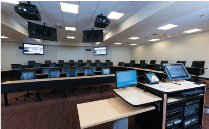
The videoconferencing system is easily activated and controlled from the lectern using an Extron TLP Pro TouchLink® Pro Touchpanel.
